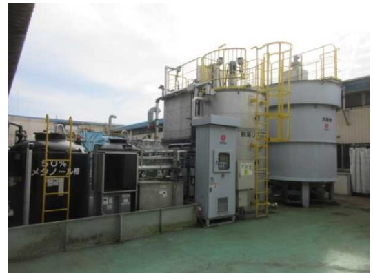
Moka Plant: biological denitrification wastewater treatment
