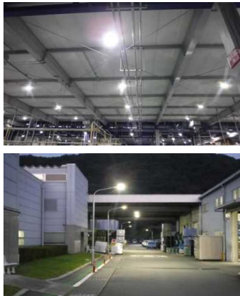
LED lighting in the premises
